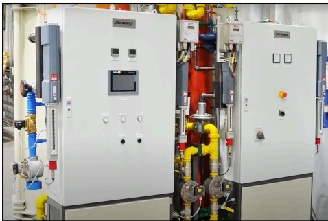
Figure 7 – Endothermic Gas Generator
