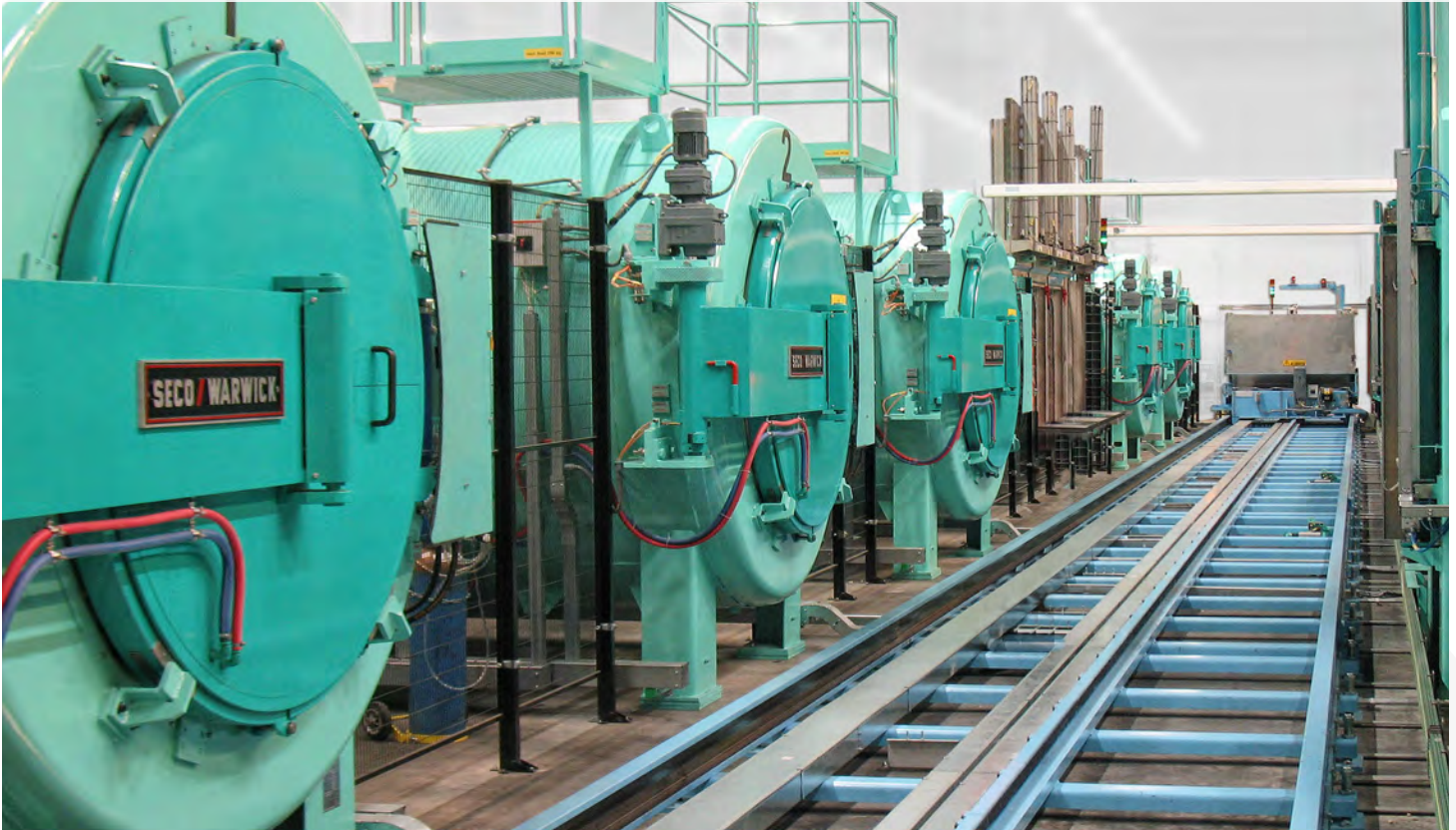
Figure 1: Nitrocarburizing system consisting of six retort-style batch furnaces
