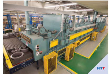
Figure 8: Cooling tunnel and exit of continuous roller hearth furnace for instrument transformer electrical steels annealing.
